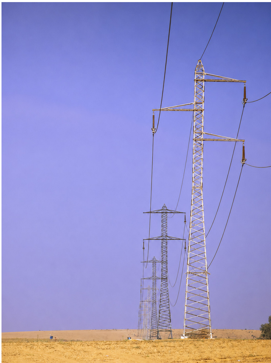
Transmission lines in the Negev, near Nahal HaBesor. Photograph: Oren Peles, PikiWiki via Wikipedia, under Creative Commons CC BY 2.5.
