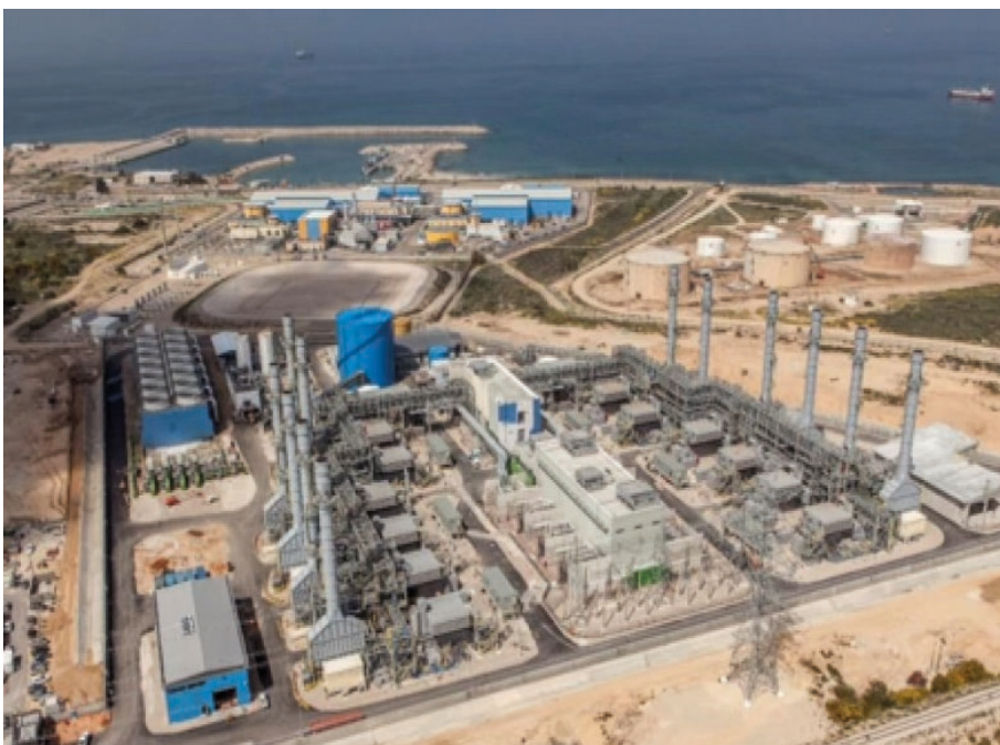
Edeltech's Dorad power station, south of Ashkelon — 860 MW combined-cycle, the flagship asset in the company's 2.9 GW portfolio. Source: Edeltech.
